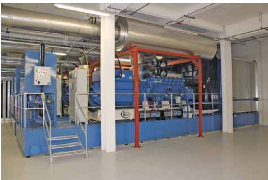
A 1 000 KVA generator set runs at around 200 litres of diesel an hour.
