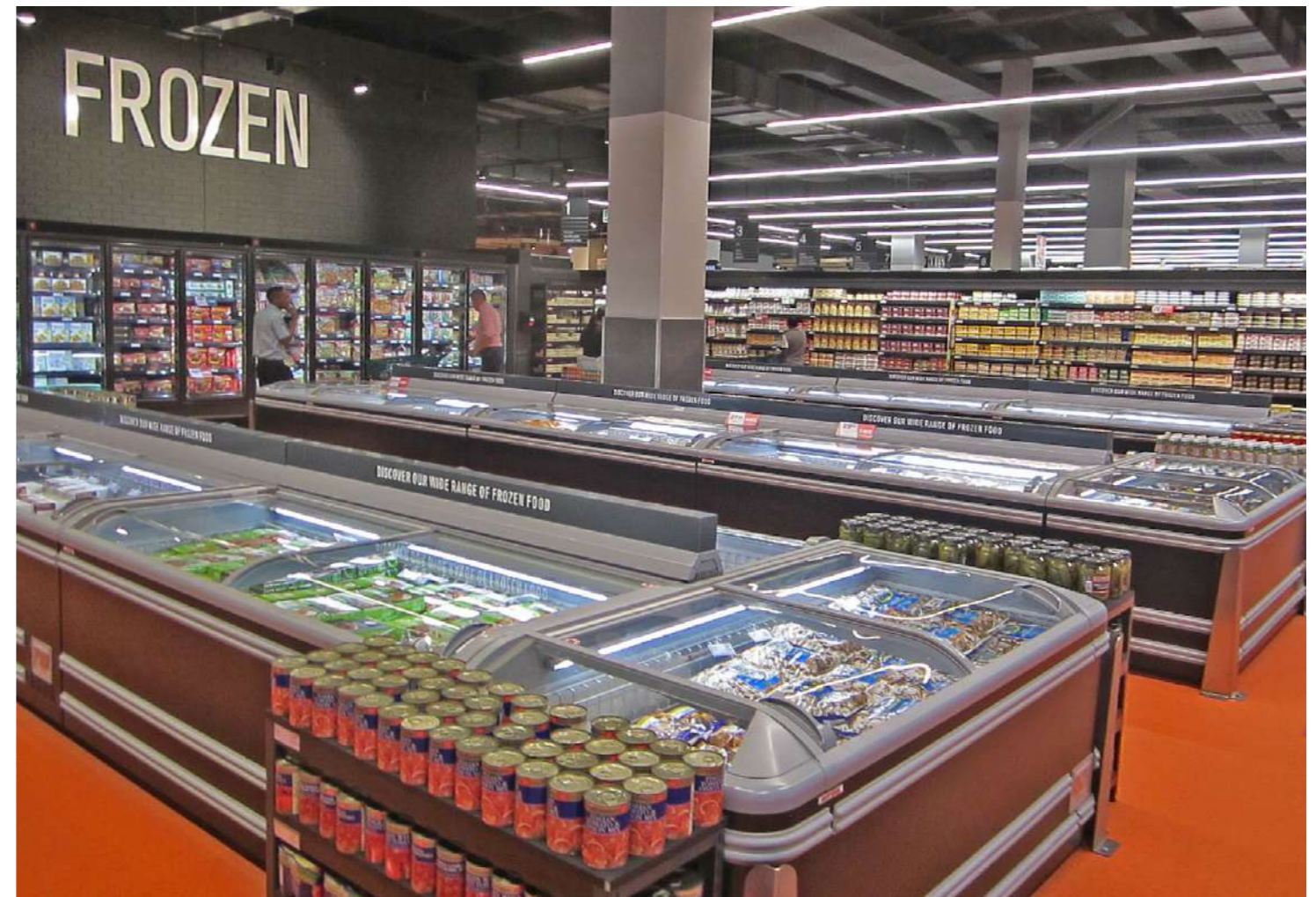
Every piece of furniture and equipment in the store has been replaced. This view shows the made-to-measure refrigeration equipment sourced from Argentina, produced to Checkers' design requirements
