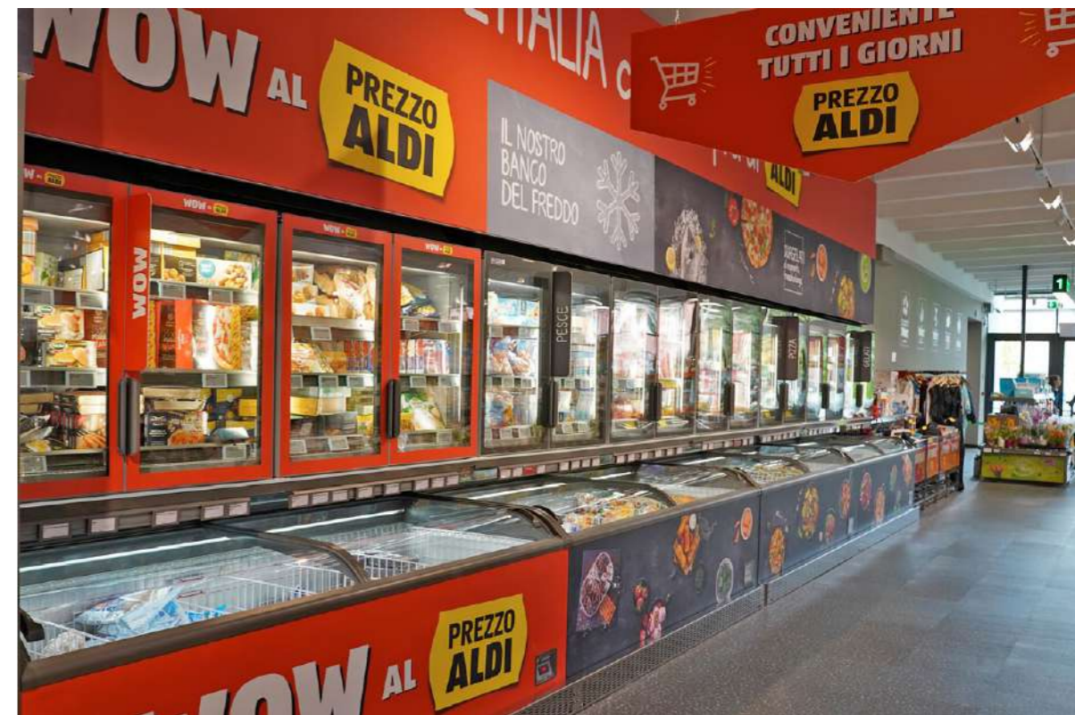
View of an aisle with frozen counters, where the bin and door combination uses the available space at its best
