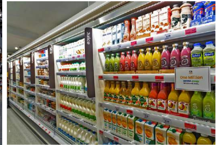
Linear display of milk and fruit juices, displayed on 'Aerofil' equipment. Sainsbury's stores are now equipped with this pioneering technology, which allows a 15% reduction in energy from its refrigerators: a sophisticated technical device in fact prevents cold air from leaving the counter, directing it back into the refrigerator.
